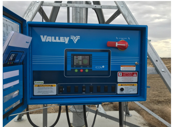
Figure 3. Control panel for a centre pivot system.
